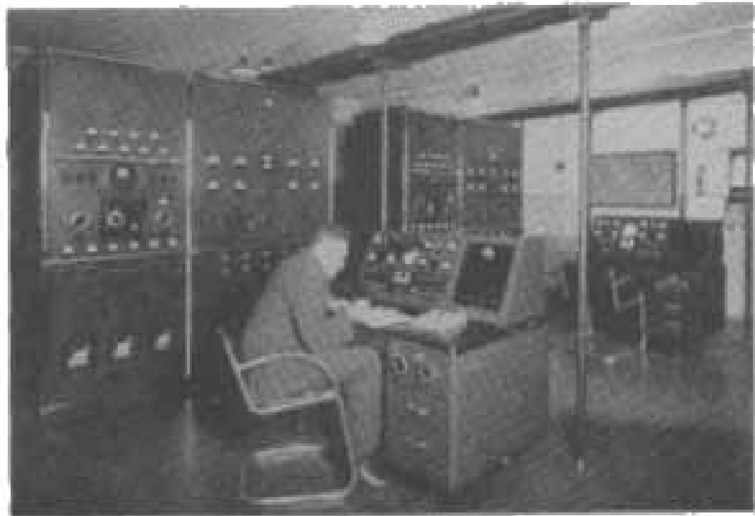
Fig. 9. East Coast CH transmitter room
